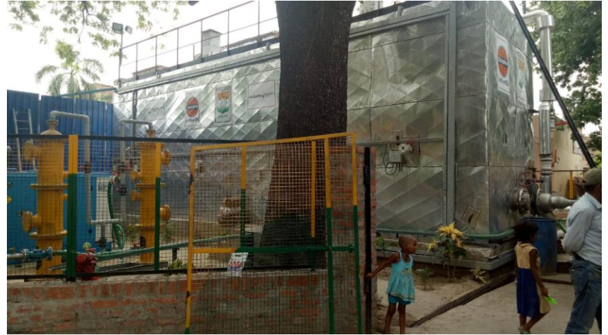
IDH Kjjakpura 5 TPD Plant
